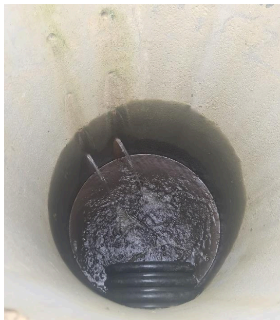
Figure 32: Paired inlet holes every 200 mm are visible with exit pipe at the bottom of the riser pipe
