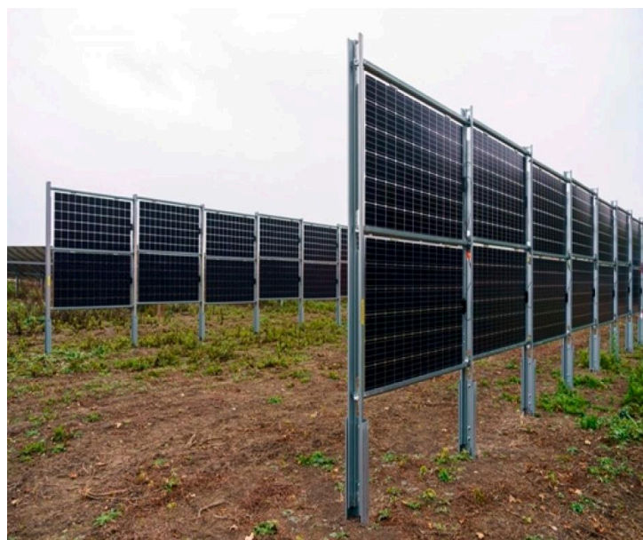
Figure 5. Next2Sun vertical system in Guntramsdorf, Austria (Toledo & Scognamiglio, 2021).
