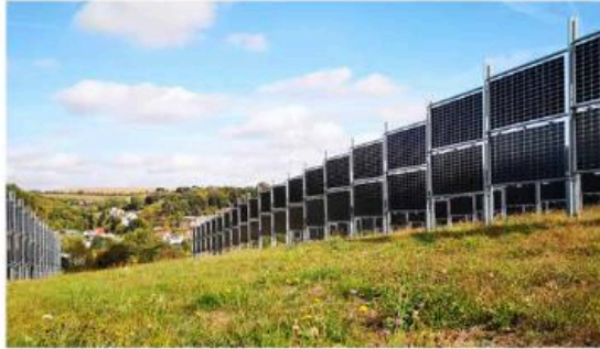
Figure 35: Bifacial modules installed vertically, Donaueschingen. © Next2Sun GmbH
